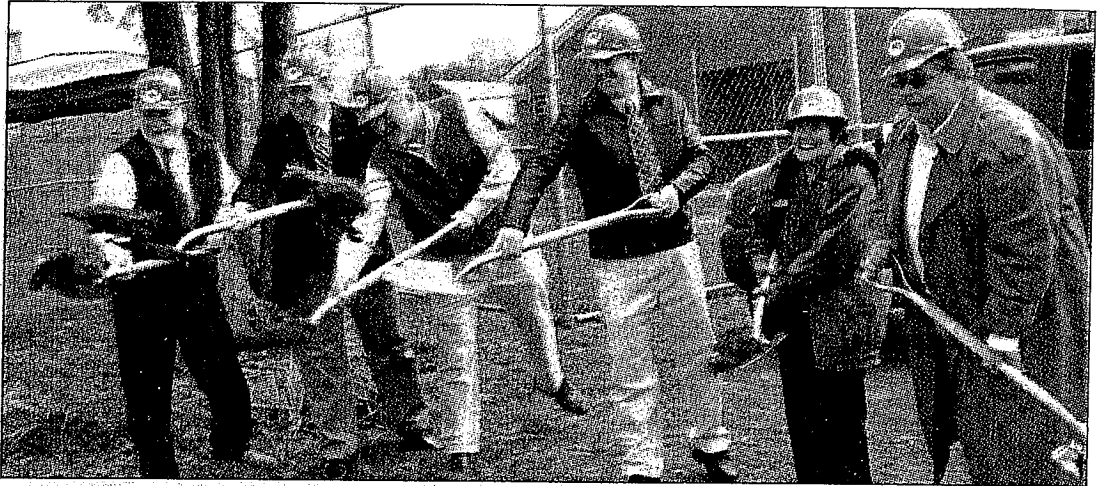
Groundbreaking ceremonies Tuesday signaled the official start of construction of the Community Corrections Center at the Sullivan County complex in Unity. From left, John Beaver, project manager of North Branch Construction of Concord, Sullivan County corrections superintendent Ross Cunningham, County Administrator Greg Chanis, Jeff Barrette, Sullivan County Commission chairman, commissioner Ethel Jarvis and State Rep. Ray Gagnon, chairman of the Sullivan County Delegation. (Archie Mountain photo)
